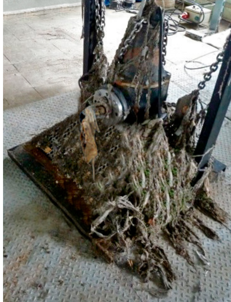
Example of clogged pump as a result of inadequate screenings removal.
